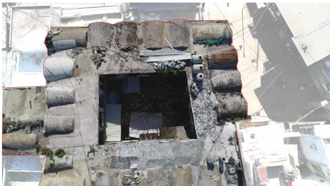
Roof extension of the Khan (original Mamluk structure from \pm 1320 ) (drone photo 3.19)
